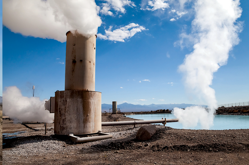
Figure 22. Dixie Valley geothermal plant. Photograph by Bridget Ayling.
